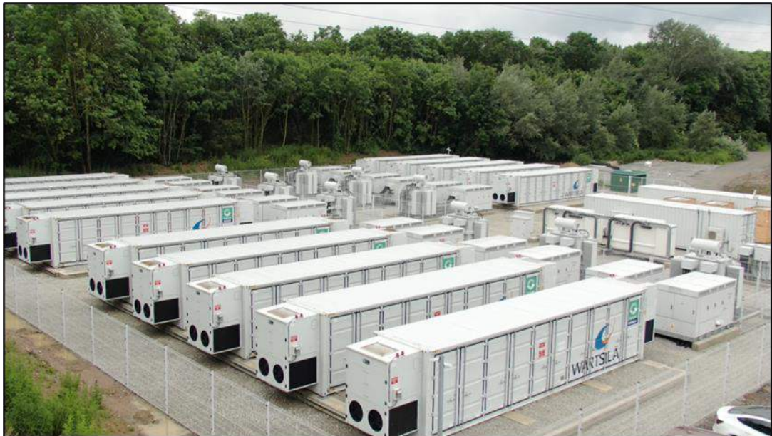
Figure 2-4: Example BESS facility
